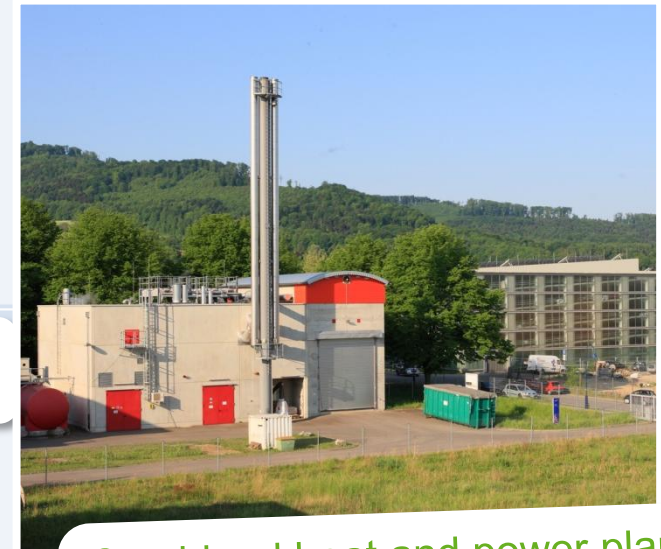
Combined heat and power plant: heat and power for the entire district of Vauban
