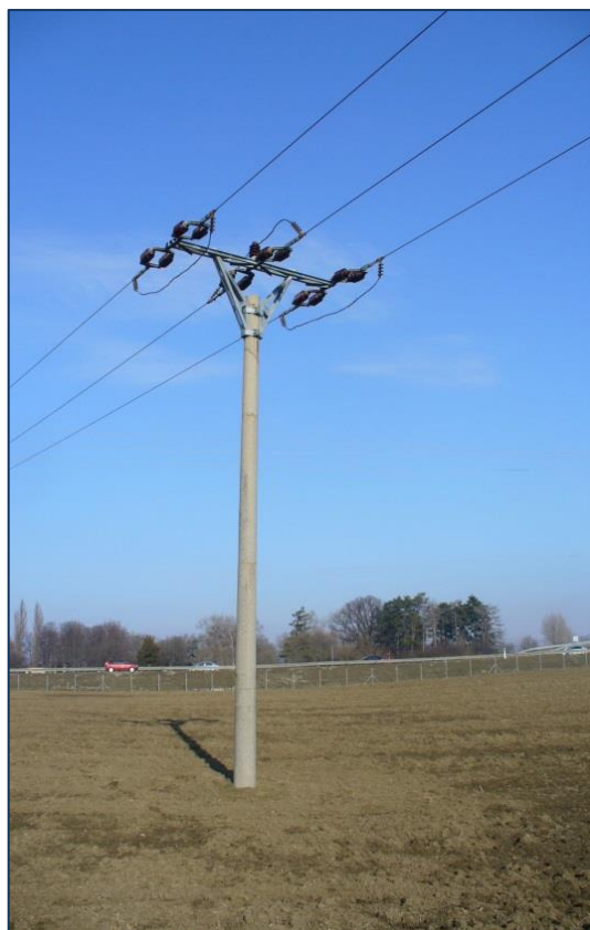
Fig. 13 Electric pole with exposed wire on the top of the console
