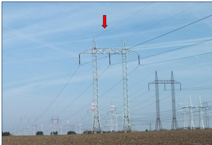
Fig. 23 The thinnest (shield) wire on the top of the power lines is almost invisible for birds
