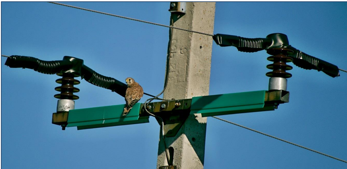
Console cover and plastic black hood on support insulator in Hungary
