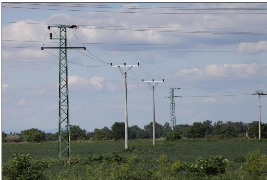
Fig. 3 22 kV distribution power line
