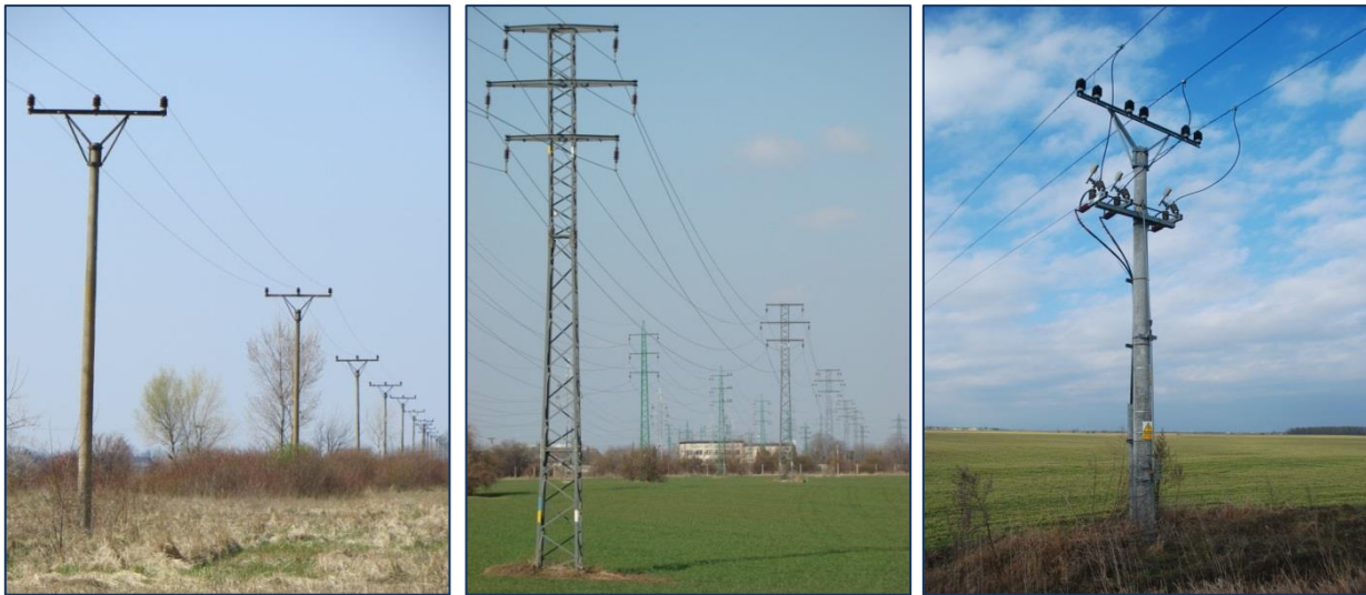
Utility poles of 22 kV line in Slovakia
