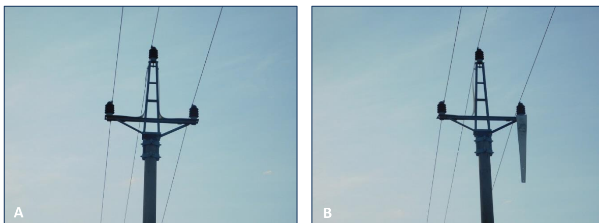
Fig. 15 Delta variant of console – good status (A) and (B) damaged status
