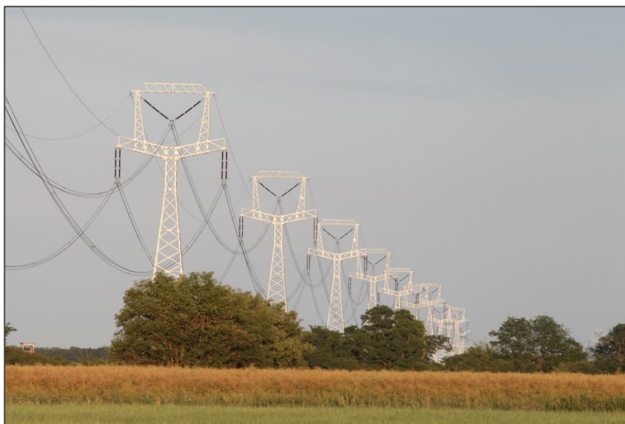
Fig. 2 400 kV transmission power line
