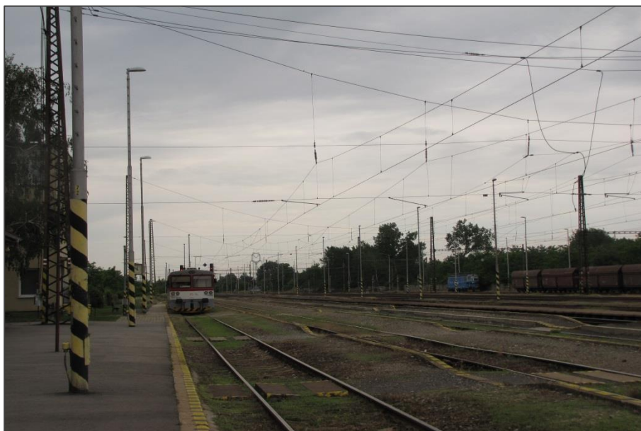
Fig. 5 Electric railway power lines
