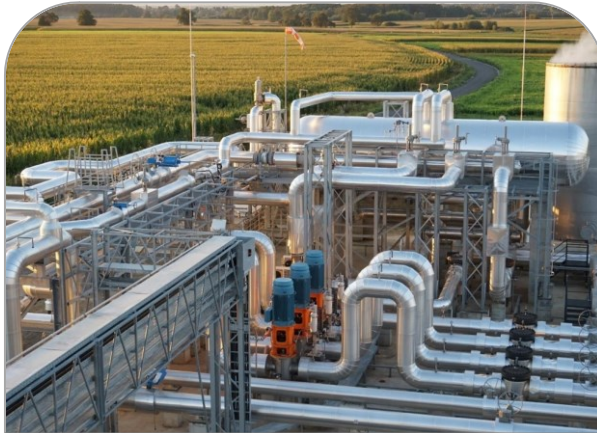
Velika Ciglena, Croatia Geothermal Power Plant
